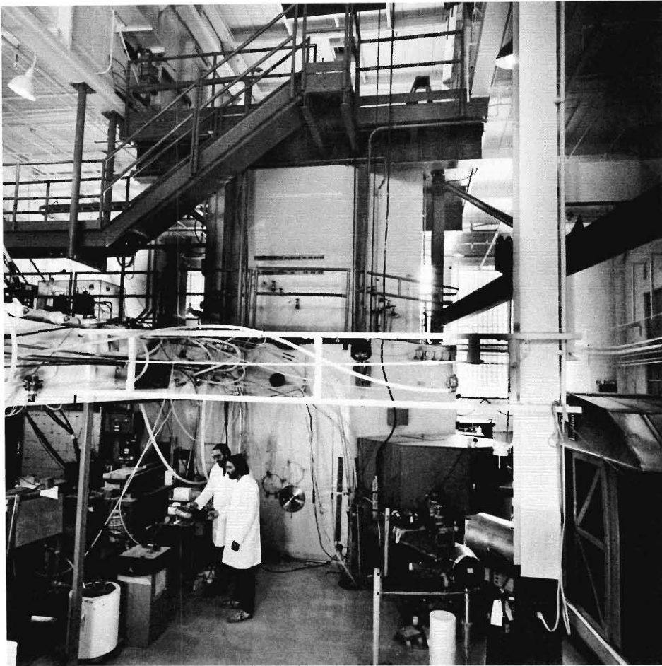
Fig. 7. North face of the Omega West Reactor. The numerous tubes above and behind the two employees are associated with automated neutron-activation analysis facilities.
