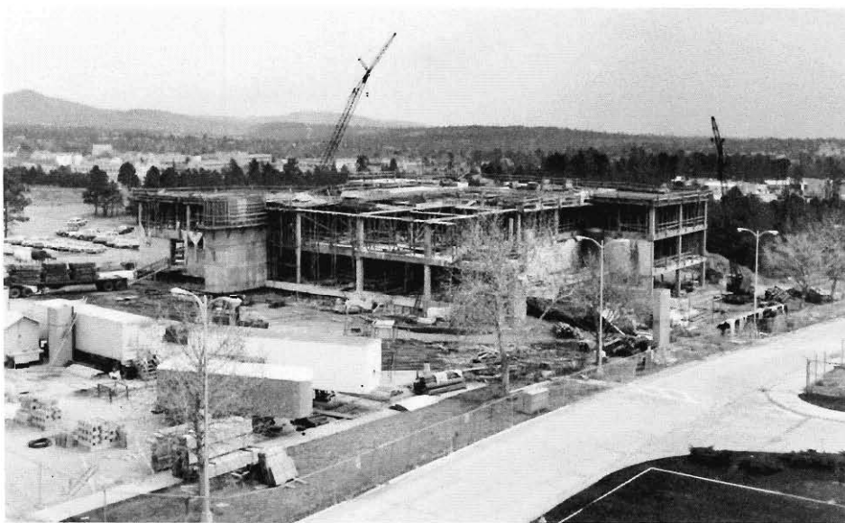
The Helios facility was constructed during the mid '70s to further explore the use of the CO 2 laser as a driver for inertial confinement fusion. Helios is an eight-beam system with an output of 10 kilojoules in 1 nanosecond.
